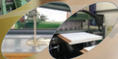
This is our panel forming plant at Peterlee. All 103 metres of it. The only one in the UK and capable of forming panel at 6 metres a minute.
